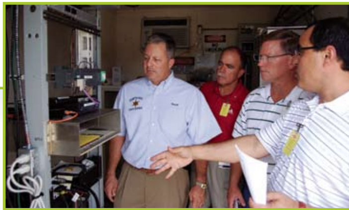
Sheriff Waguespack and officials from the Louisiana Department of Public Safety examine the electronics of the new radio system at the tower site.
